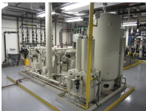
Medical air compressors
