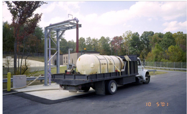
Figure 5-14 Cary, N.C., bulk fill station allows approved contractors, landscapers, and town staff to use reclaimed water
