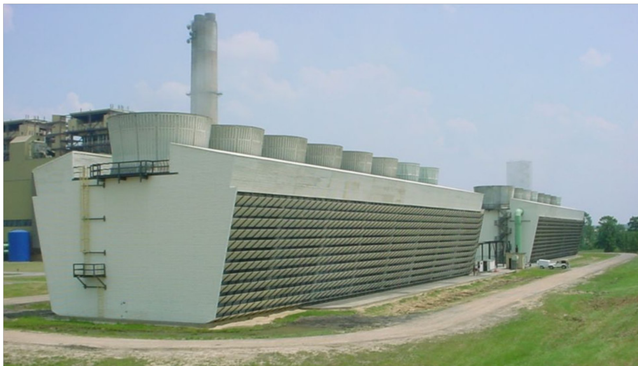
Figure 3-5 Large hyperbolic cooling towers (Photo Courtesy of International Cooling Towers)
