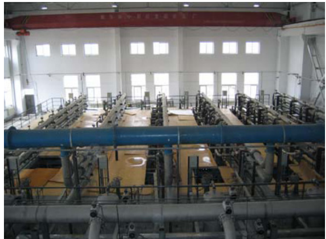
Figure 1 Hohhot MBR facility (Photo credit: Courtesy of GE Water and Process Technologies)
