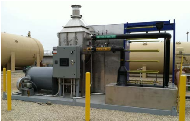
Figure 1 400 gpm Wastewater Pasteurization Demonstration System in Ventura California (Photo credit: Greg Ryan, Pasteurization Technology Group)
