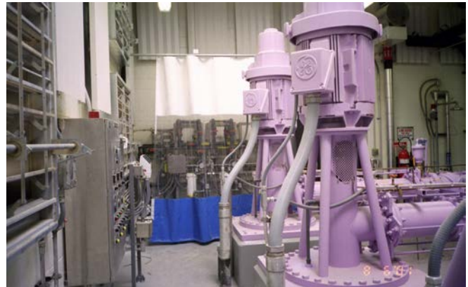
Figure 2 New reclaimed water pumps at the WRF (Photo credit: David Heiser)
